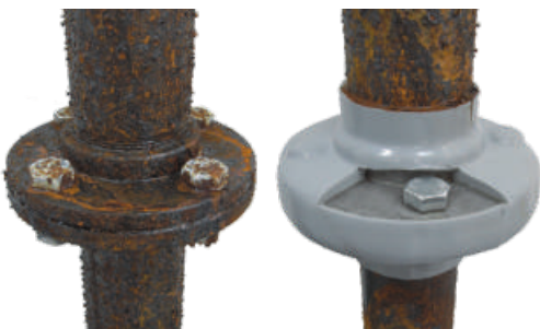
Unprotected corroded flange - Successful protection with Oxifree TM198
