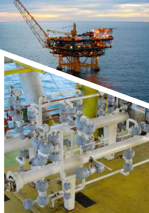
OFFSHORE APPLICATIONS An average of 45 to 55 flanges were coated per day making this a very cost effective operation
